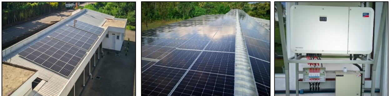
Picture 5: Pictures of 500 kW Solar Roof Top Power Plant in UTP, Mawathagama
