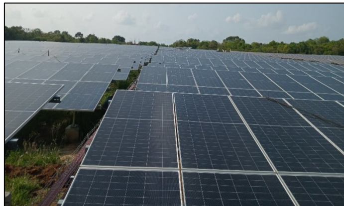
Picture 2: Pictures of 10 MW Solar Power Plant in Kebithigollewa
