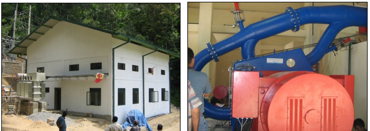
Figure 7: Pictures of 2MW Mini Hydro Plant in Aranayaka
