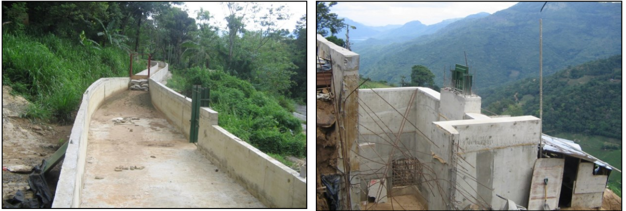
Figure 8: Pictures of 2MW Mini Hydro Plant in Walapane
