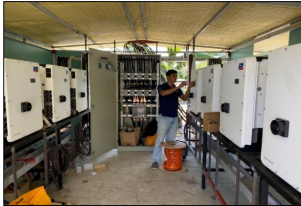
Picture 4: Pictures of 550 kW Solar Roof Top Power Plant in Embilipitiya
